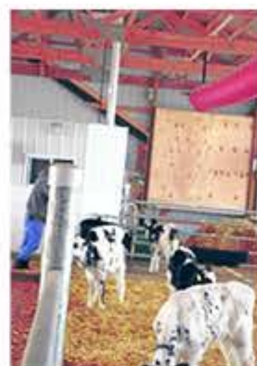
Plywood boxes cover exhaust fans located about 4 feet off the floor to draw up stale air from the lower 3 to 4 feet of the barn — the area where calves breathe.
