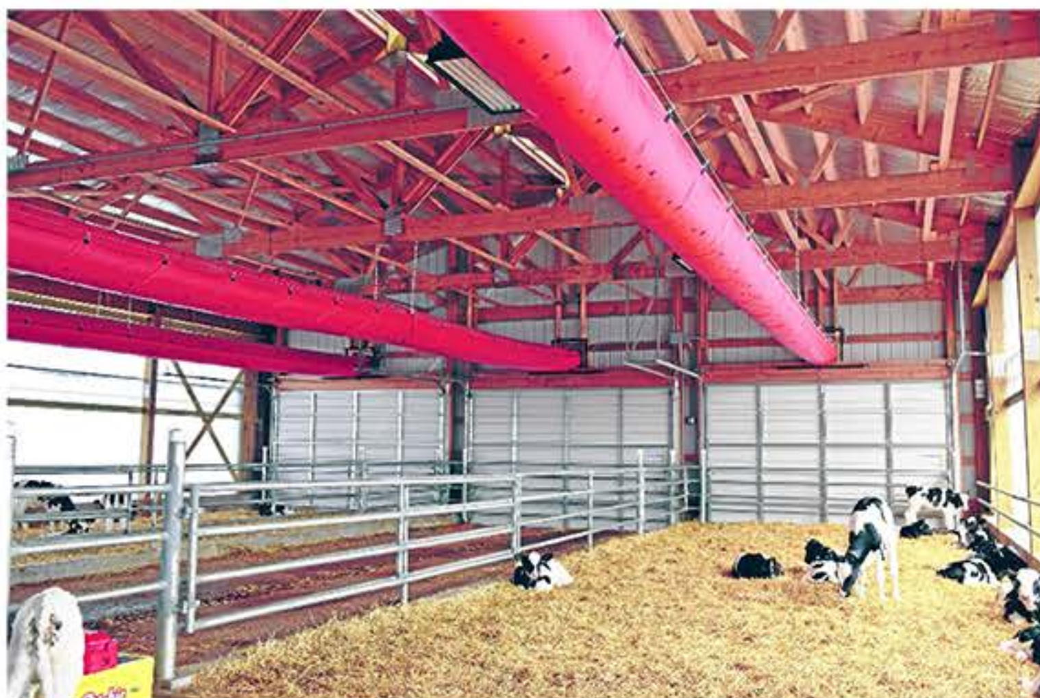
Mighty Grand Dairy's new calf barn positive-pressure ventilation system was developed by Dr. Ryan Leiterman, a veterinarian and director of technical services at Crystal Creek Veterinary Service in Spooner, Wisconsin.
