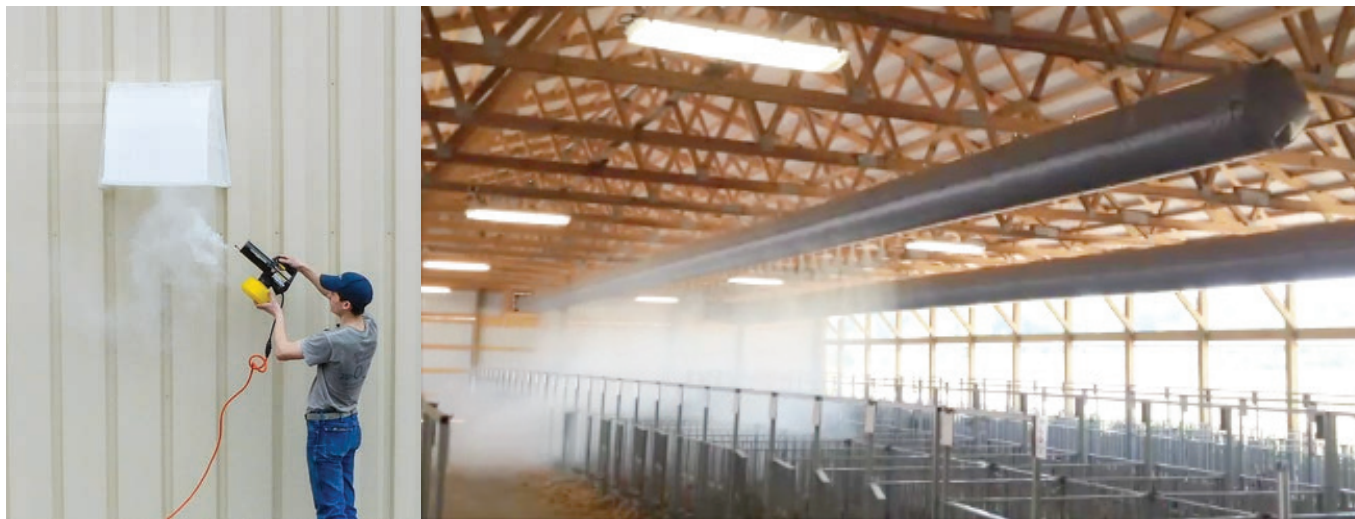
FIGURE 3 Introducing fog next to the intake of an outside fan will demonstrate the path outside air takes once it enters the barn
