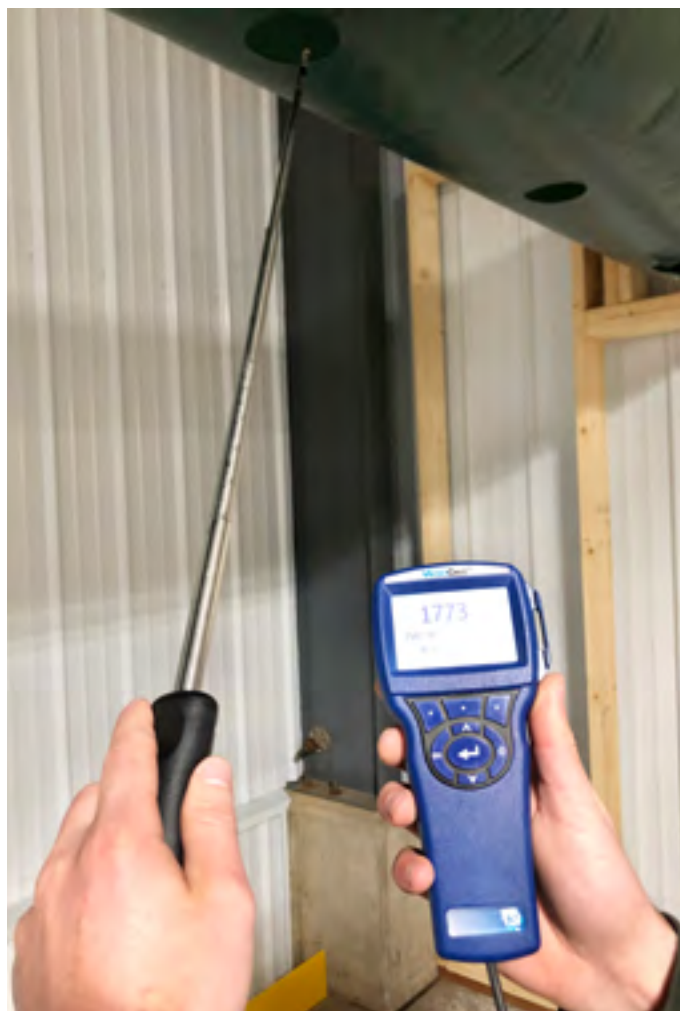
Picture 1: A hot wire style air speed meter is used to measure air speed and volume from a positive pressure tube.
